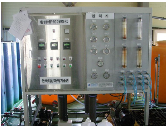
Fig. 2. NF/RO 3 modules desalination system for mineral control installed in the Deep Ocean Water Research Center (DOWRC) of Korea Institute of Ocean Science & Technology (KIOST).
