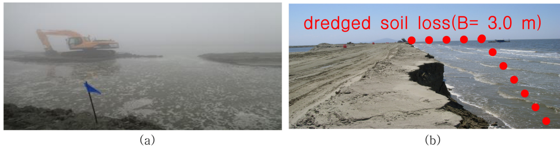
Fig. 3. (a) An inundated construction equipment and (b) a washed catch canal drain away.
